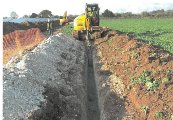
Cable trenching, showing topsoil stripped and set to one side, with subsoil placed on the other side ready for reinstatement (photo courtesy of British Solar Renewables)
